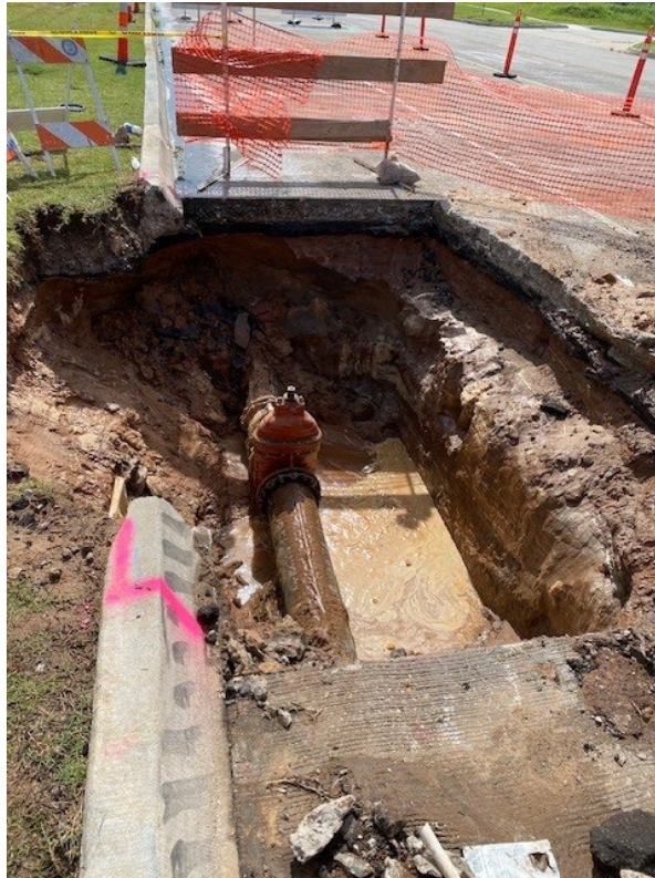
FIGURE 2 – 12" GATE VALVE INSTALLED
